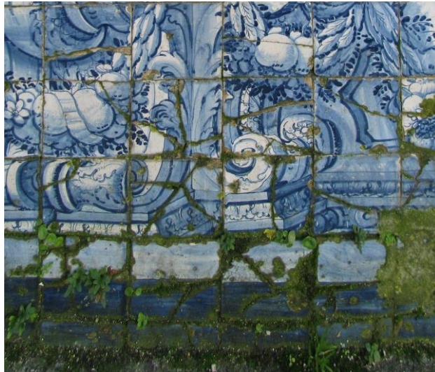
Figure 1- Decaying panel in a now exposed area (Oporto Cathedral, upper cloister gallery)
