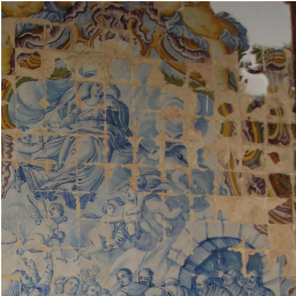
Figure 4- Generalized decay at the wet zone of an interior panel (Church of Jesus, Setubal)
