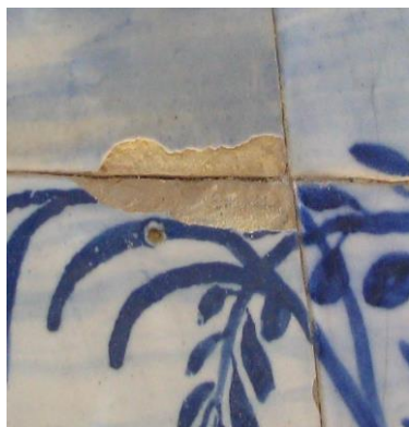
Figure 5 - Decay progressing from edges
