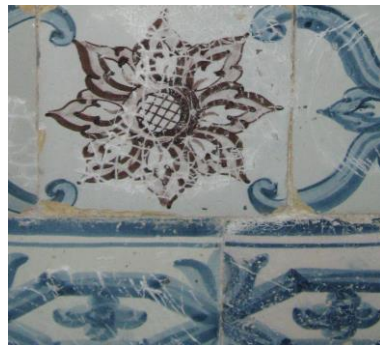
Figure 3b- Efflorescence at the same panel
