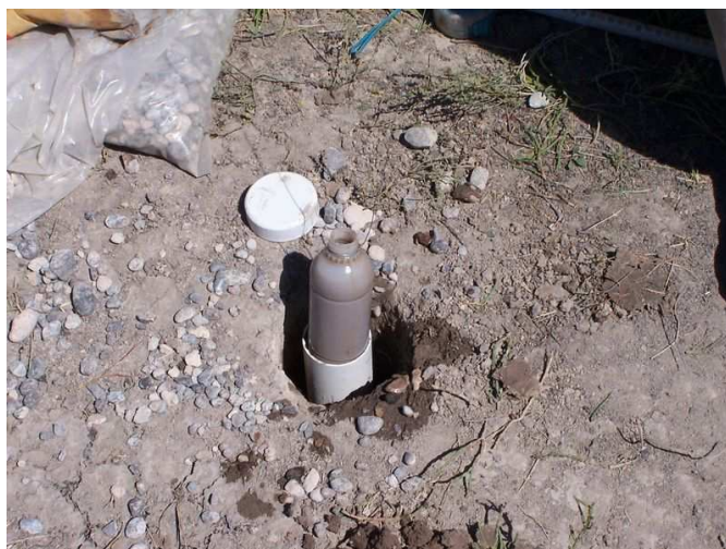
Fig. 8 - Piezometer installed for ECOMANAGE project
