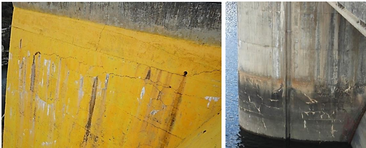
Figure 1.4: Map cracking at the top of the left abutment (left image) and on the right surface of pier 1D, upstream (right image) (photos taken in June 2019)
