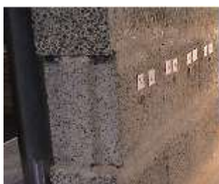
Fig. 15: Aspect of the Specimen A2 in the compression test, with signs of slight surface cracking in mortar joints
