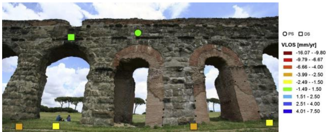
Figure 72 – Improved location of PSs (circles) and DSs (squares) on an aqueduct aided by RTK GPS observations; colours correspond to LOS velocity (Tapete et al. , 2015).
