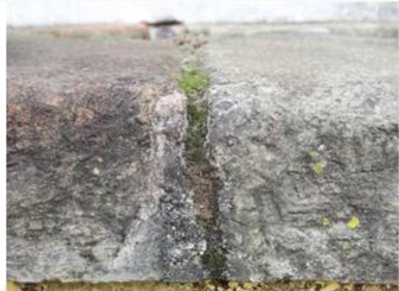
Figure 21: Colonization of moss in the joint between the stone parts of the tank: authors' file, 2021.
