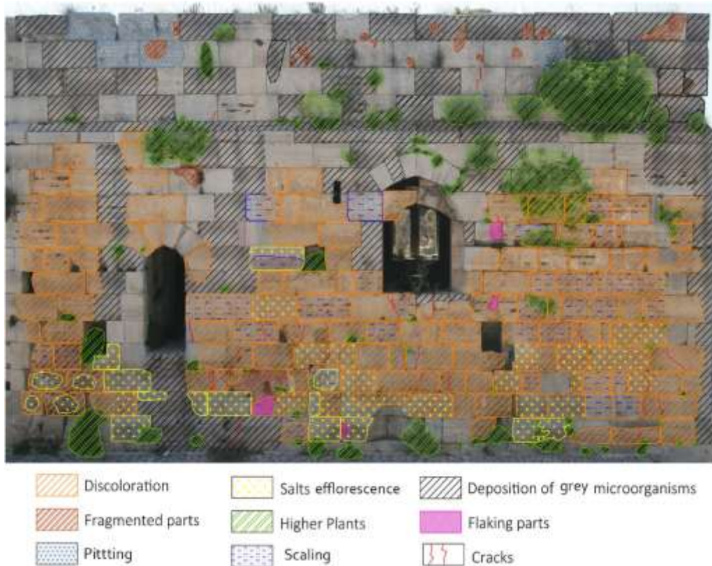
Figure 4 Deterioration mapping of the external east facade of the building (36).
