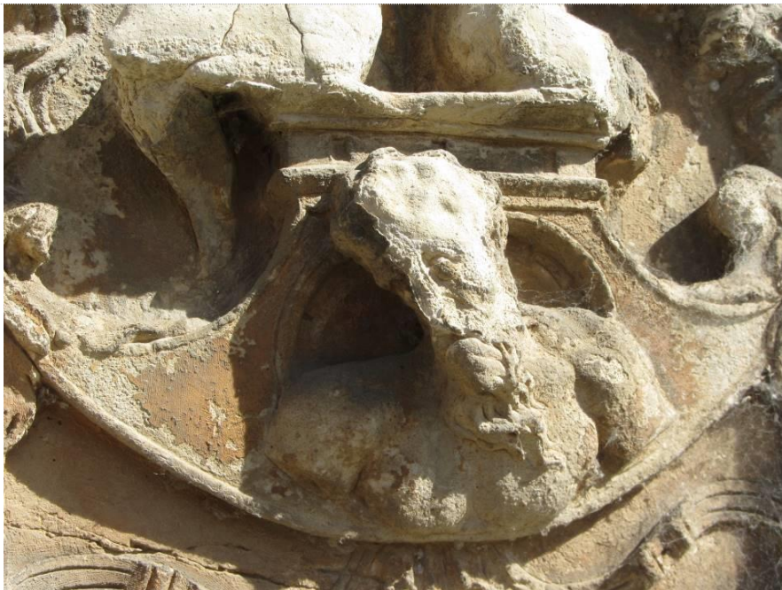
Figure 1 – A thin superficial indurated crust, possibly caused by a past consolidation treatment, often ends up failing by excessive incompatibility with the substrate, as happened in this very porous limestone
