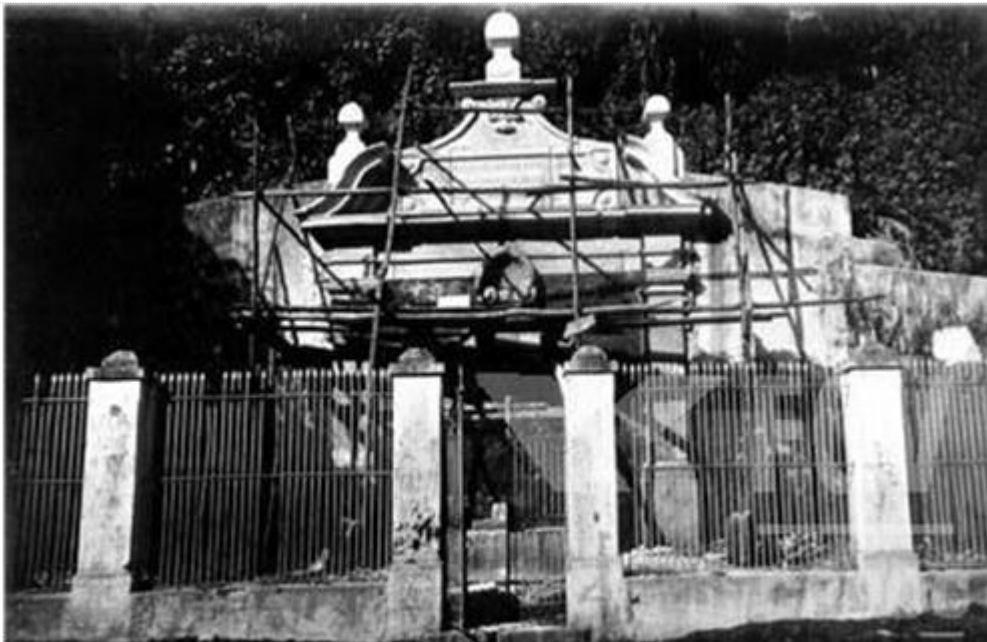
Figure 5: Restoration work at Chafariz da Glória , Ouro Preto, in 1935. Source: http://www.fgv.br/cpdoc/acervo/arquivopessoal/GC/audiovisual/aspectos-de-obras-de-restauracao-de-churches-and-monuments-made-by-the-service-of-the-historical-and-artistic-national-heritage . Accessed on February 6, 2021.
