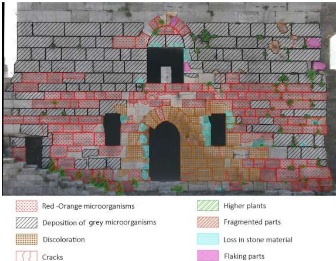
Figure 6 Deterioration mapping of the external north facade of the building (36).
