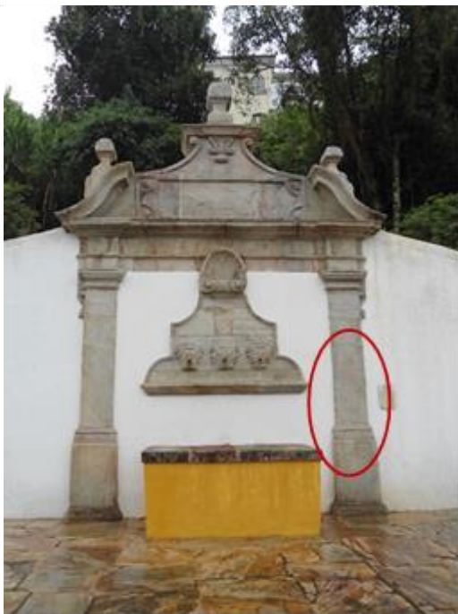
Figure 12: Photograph of the Fountain right after the restoration. Source: National Historical and Artistic Heritage Institute, 2015.
