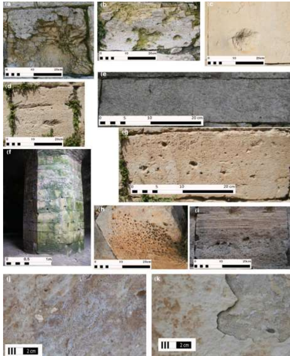
Figure 3 Deterioration cases at the castle. a) Demolished fragmented stone. b) stone exposed to missiles fragments. c) Stones exposed to a direct bullet. d) Growing of invasive plants in the joints. e) Deposition of grey microorganisms. f) Green microorganisms on a pillar exposed to water infiltration from the roof. g) Orange discoloration. h) Pitting. i) Deposition of red-orange microorganisms. j) Salt efflorescence. k) Scaling.
