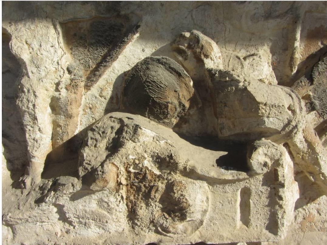
Figure 2 – Consolidation of a delicate surface showing strong signs of deterioration requires a slight increase in strength and with a very low degree of incompatibility. High-strength increments and very shallow impregnation depths, as this photo suggests, can compromise the entire surface in the medium to long term
