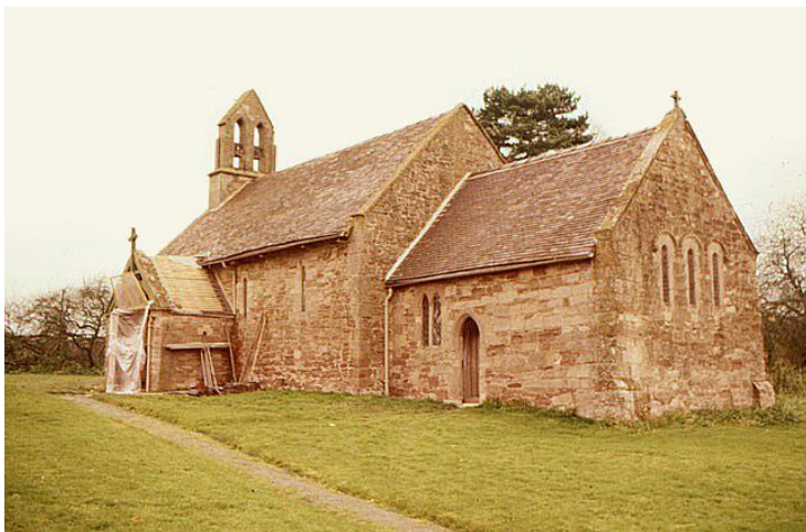
Figure 1. Aston Eyre Church showing the entrance porch containing the tympanum sheeted with protective polythene during consolidation in 1974 (photo: Deborah Carthy).
