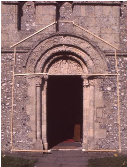
Figure 6. St Nicholas church, Barfrestone. Main doorway with carved decorative stonework framed for polythene sheeting prior to consolidation treatment in 1977 (photo: Deborah Carthy).
