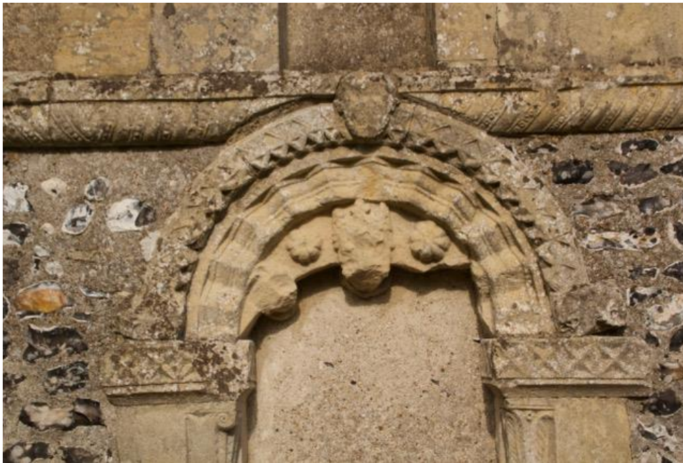
Figure 14. St Nicholas Church, Barfrestone. Extensive stone erosion and significant lichen growth on the stonework of the unconsolidated south-facing doorway in 2019 (photo: Deborah Carthy).
