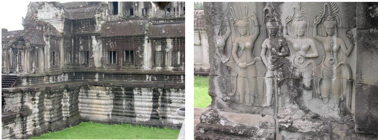
Figure 8 a + b: The removal of the natural biofilms led to an intensive regrowth of blackening cyanobacteria at Angkor Vat with additional thermal-hygic stresses to the sensible clay-containing sandstone resulting in a severe detachment of rock shales from Apsara carvings
