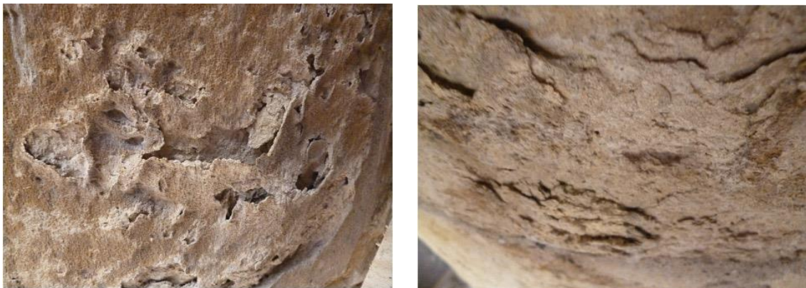
Fig. 6 Two types of degradation that are not to be treated with a consolidant; left, bulging / blistering, right, exfoliation
