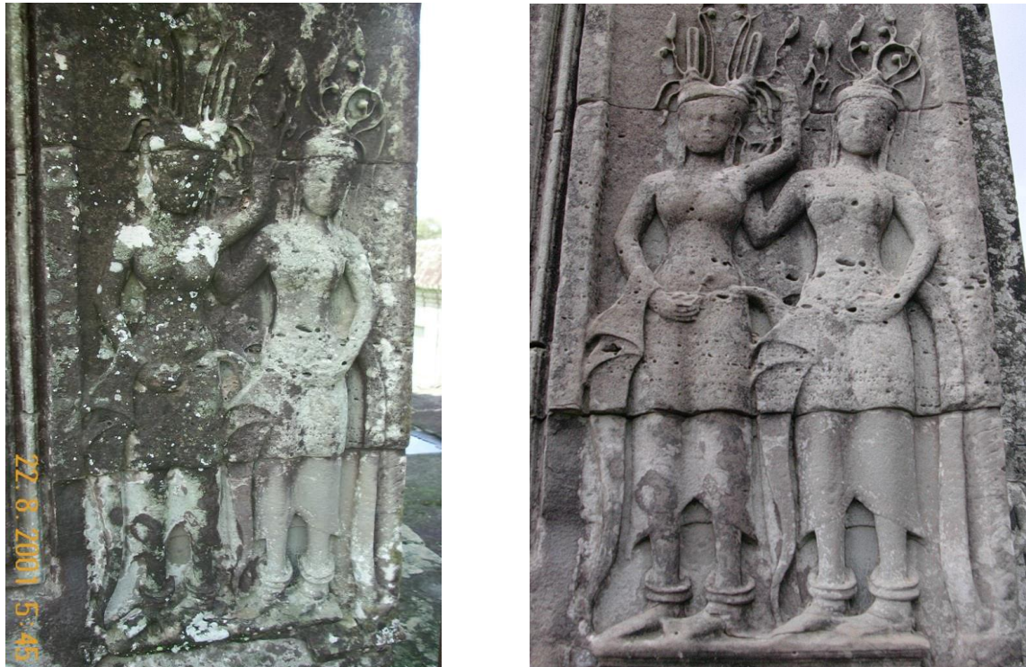
Figure 9 a + b: Successful application and long-term efficient protection of a specific designed biocidal formulation at the northern bibliotheca at the Angkor Vat within the 3rd enclosure four years after treatment.
