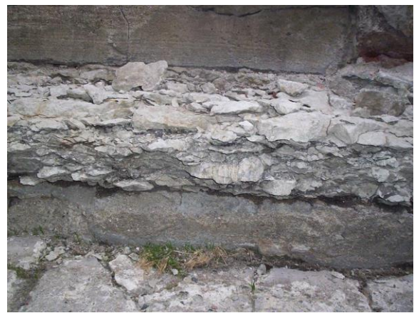
Fig.4 Crumbling of stone, photo from MDCS
