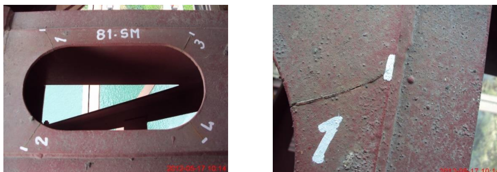
Fig. 2 – Fendas no Painel 81
