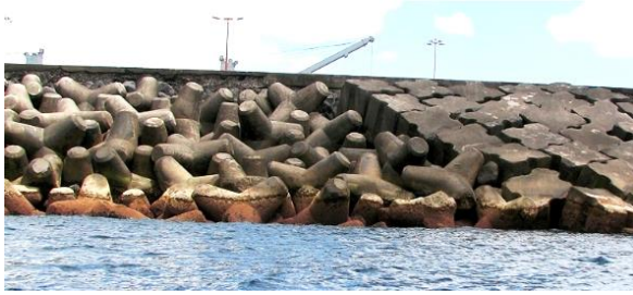
Figure 8 – The armour layer of a breakwater with two different kinds of blocks: tetrapods and Antifers
