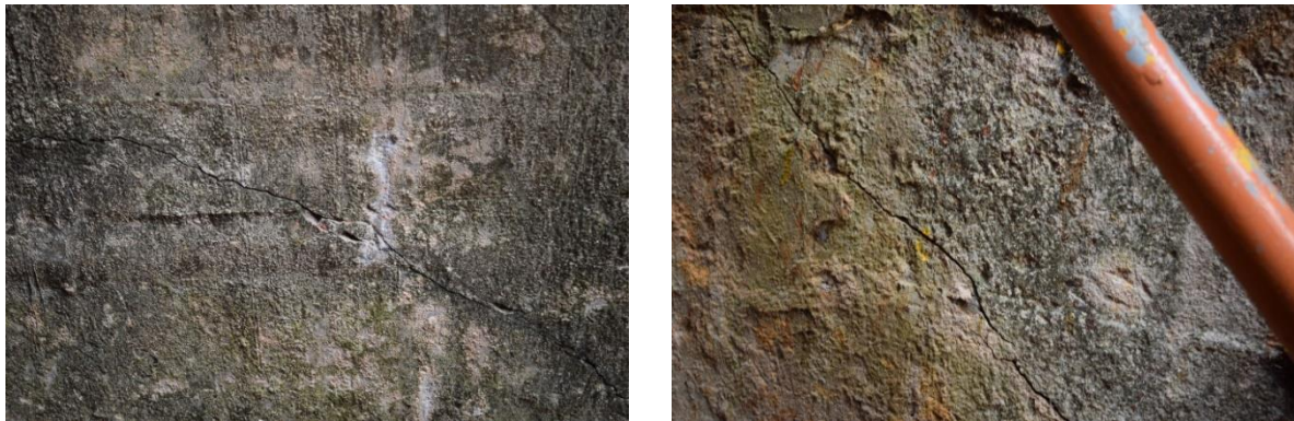
Fig. 6 – Views of cracks parallel to the dam-foundation interface, on the downstream surface of the secondary arch, on the right bank side, between joint II and the middle of block IV-V
