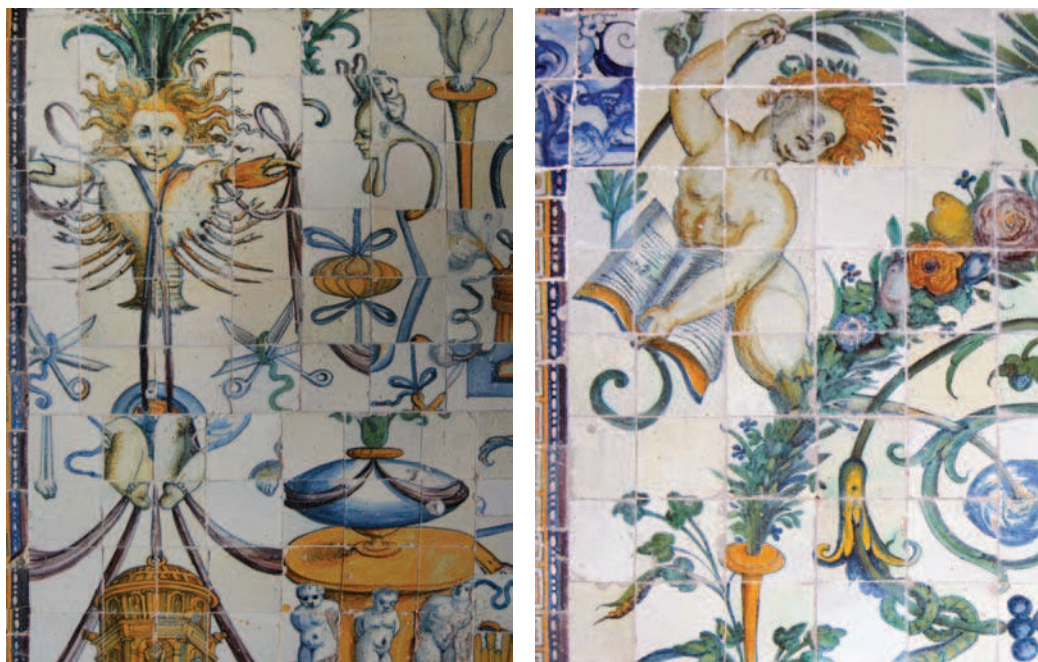
Figure 1. Two aspects of the azulejo panels in Graça church from where samples Az013 were collected
