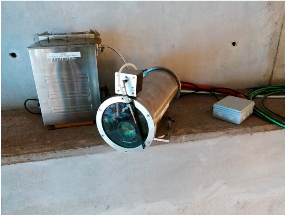
Fig. 3. Camera assembly on one of the beams.
