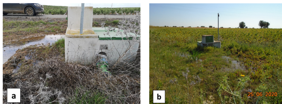
Figure 25. Pictures of hydrant H9.18 and surrounding vegetated ground taken on (a) 16 April 2020 and (b) 25 June 2020.
