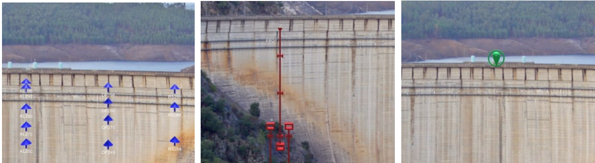
(a) Geodetic marks (b) Plumblines (c) GNSS
