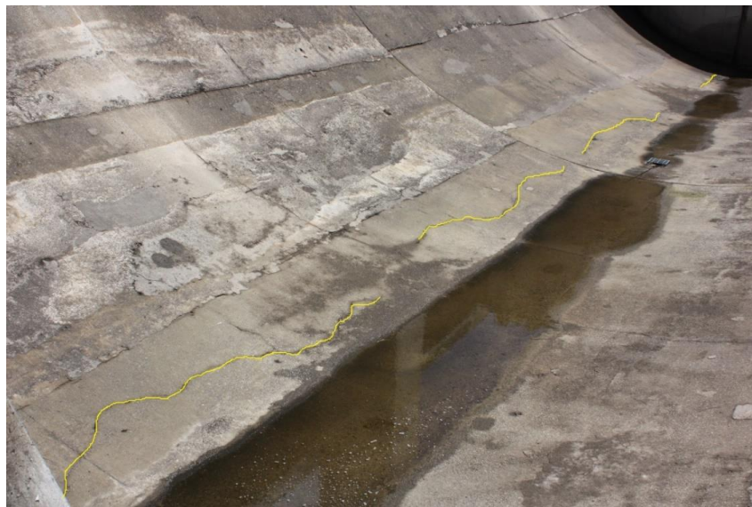
Figure 15: Stabilized longitudinal crack on the ski jump bucket
