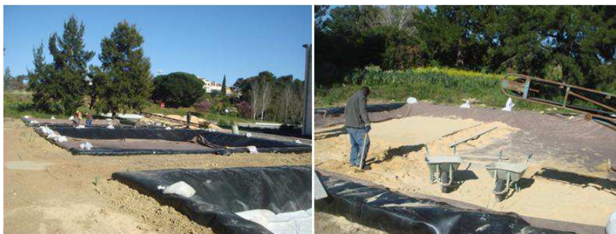
Figure 1 Pilot cells construction at LNEC's campus. Right photo – detail of drainage layer (sand) installation.
