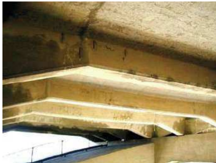
Figure 1. – Carbonation and the corrosion of the reinforcement (source: Duratinet).
