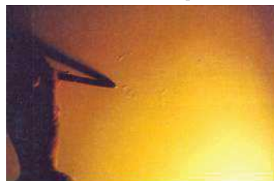
Blistering in "plastic paint"
