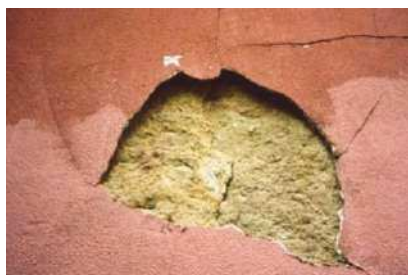
Figure 5. – Blistering and detachment of the render.
