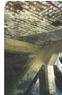
Figure 2. – Corrosion due to chloride ingress (source: Duratinet).
