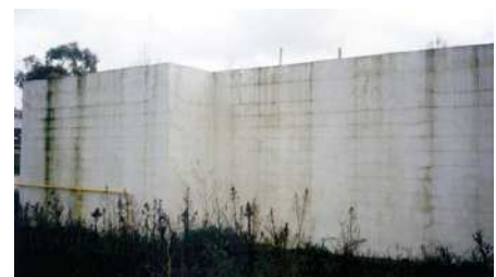
Figure 7. – Horizontal cracking following the joints.
