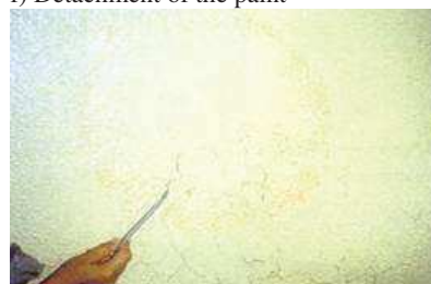
h) Cracking in "Kerapas" type paint
