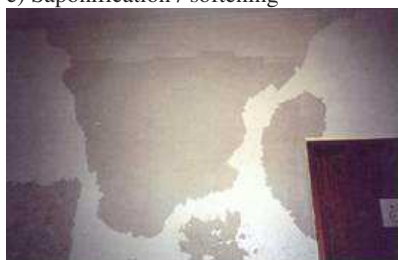
g) Detachment of the paint
