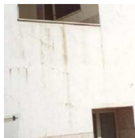
Figure 6. – Mapped cracking due to shrinkage and efflorescence's.
