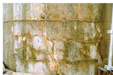
Figure 4. – Alkali aggregate reaction (source: Duratinet).
