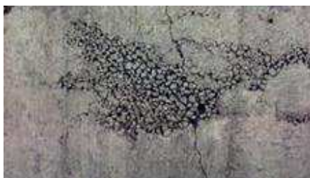
Figure 3. – Freeze thaw deterioration.
