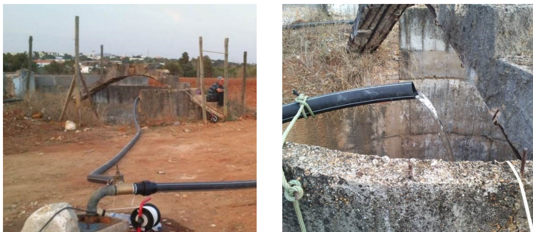
Figure 57 – Infiltration test at DEMO site PT1_3, injection test at a large diameter well. The pumping well can be seen on the bottom of the left picture
