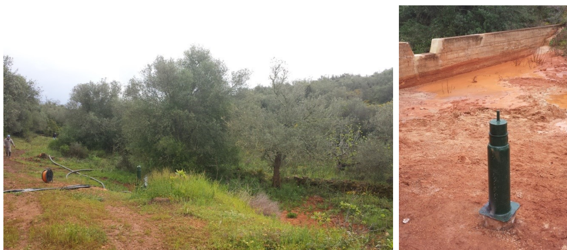
Figure 77 – New piezometers at Cerro do Bardo. CB1 in the left and CB2 in the right
