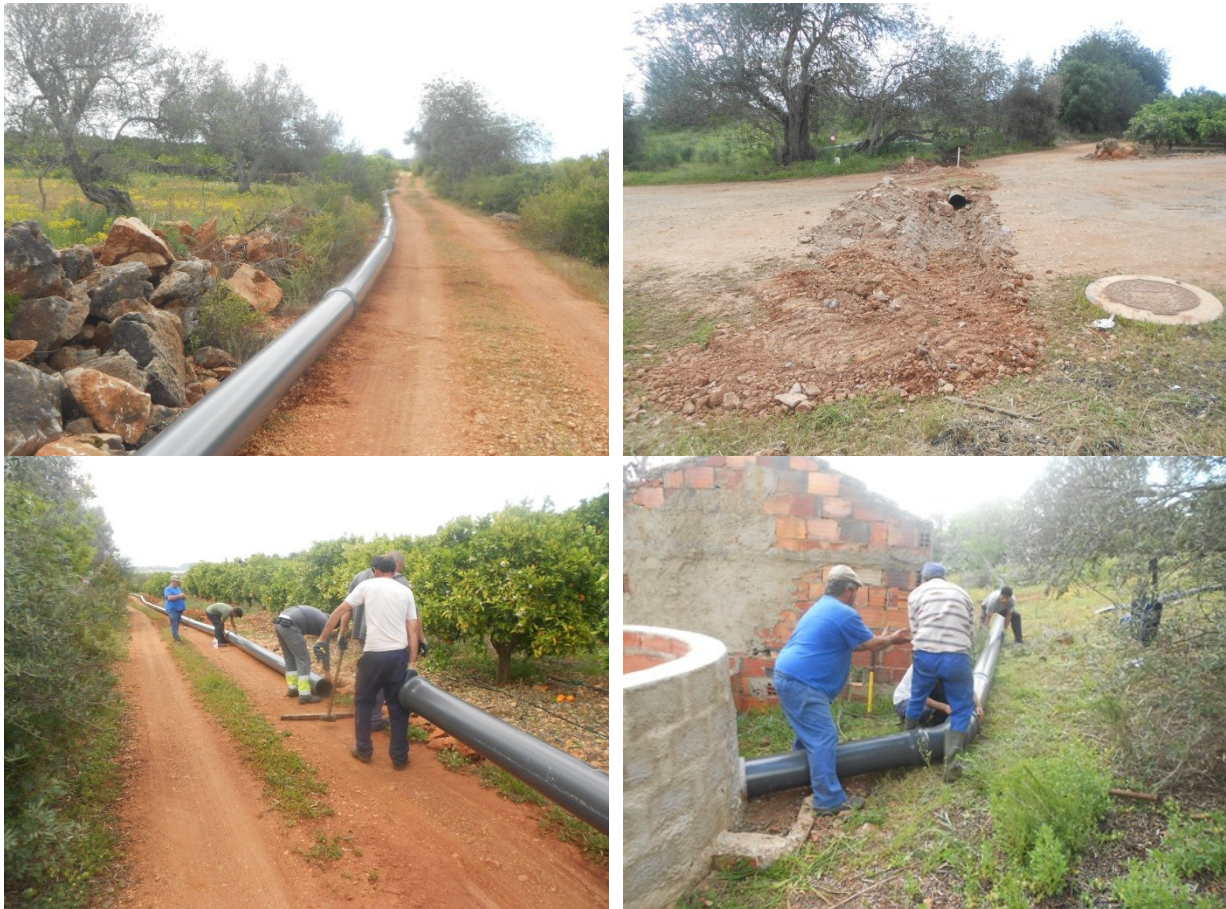
Figure 120 – Illustration of the work to install the 1.4 km pipeline from SJS2 well to CB well
