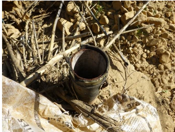
Figure 8 – LNEC2 piezometer without ladle
