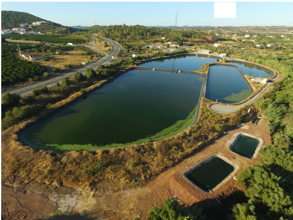
Figure 71 – MARSOL SAT basins at S. Bartolomeu de Messines waste water treatment plant
