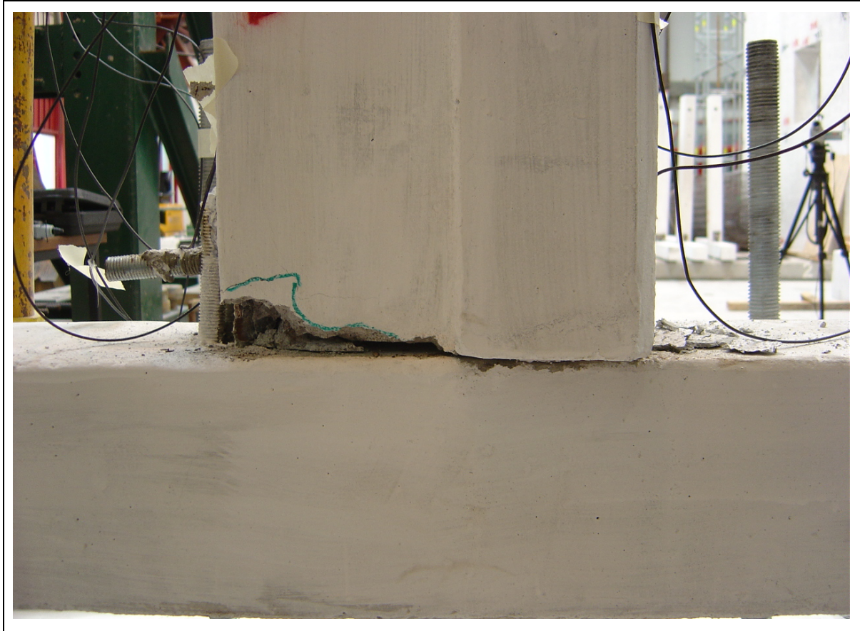
Figure C.29: Specimen VL1 – View of the initial damage.
