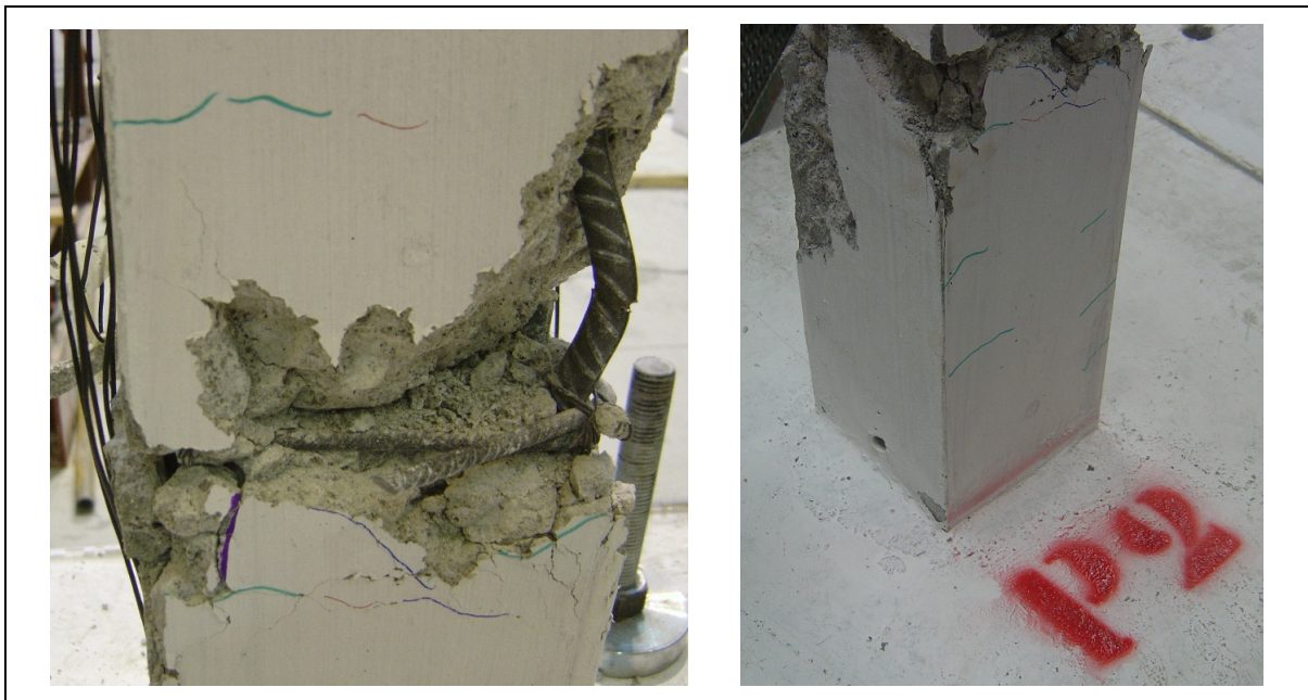
Figure C.8: Sp.P2 – Detail of the collapse zone and of the column-foundation connection.
