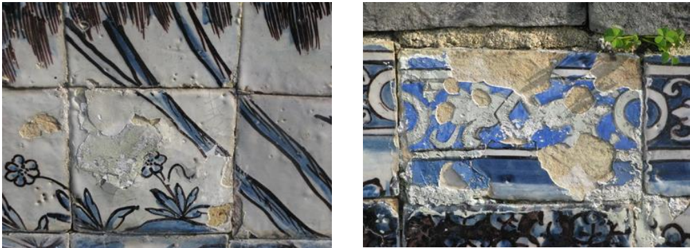
Figure 1. Lacunae infill treatments with issues of lack of compatibility, efficiency or durability. Palácio Fronteira, Lisbon, 2012. Photos by S. Pereira
