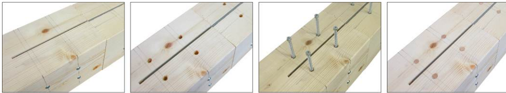
Figure 7: Reinforcement with self-drilling screws: unreinforced connection, boring the clearance holes, driving the screws, and inserting the wooden plugs (connection D05.1)
