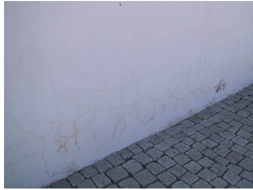
Fig. 15 - Cracking of render/paint system (2002-07-03)
