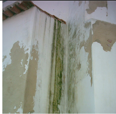
Fig.22 - Water flow marks from the tiled roof and biological growth (2003-11-19)
