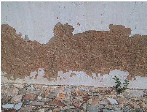
Fig. 16 - Detachment of paint and cracking of render (2003-10-30)
