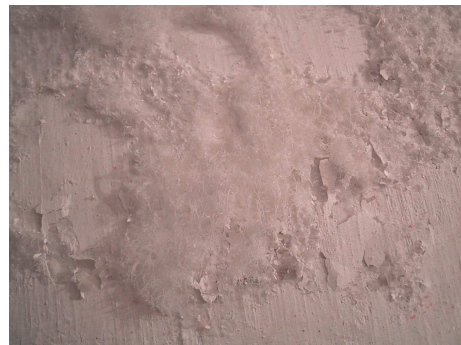
Fig. 24 - Efflorescences and detachment of paint on an internal wall (2002-07-03)
