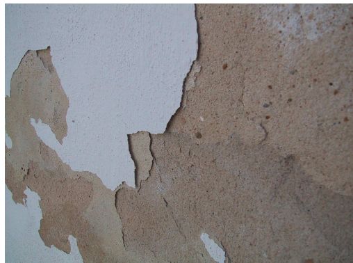
Fig. 19 - Detachment of paint and of render superficial coat (2002-07-03)
