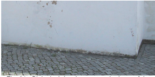
Fig. 21 - Biological development at the base of the northern façade (2003-11-19)
