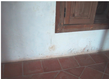
Fig. 25 - Efflorescences, detachment of paint and sanding of render at the base of an internal wall (2003-10-30)
