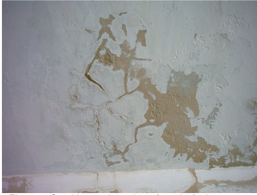
Fig. 14 - Cracking and erosion of render/paint system (2003-11-19)
