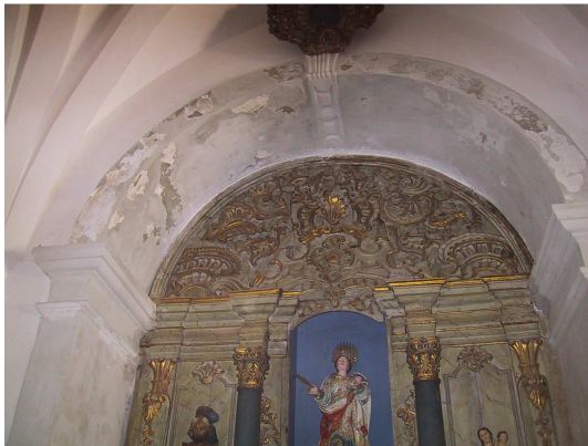
Fig.23 - Detachment of paint at the interior of the church (2002-07-03)
