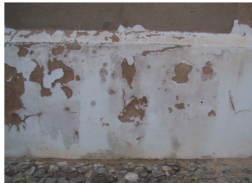
Fig. 20 - Moisture spots and other degradation of render/paint system (2003-10-30)
