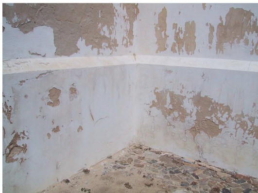
Fig. 12 - Sanding of render and crumbling of render/paint system (2002-07-03)
