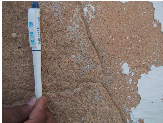
Fig. 17 - Cracking of render (2003-10-30)
