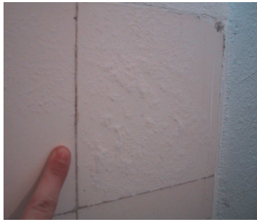
Fig. 22 – Efflorescences on the WC ceramic tiles (2004-01-06)
