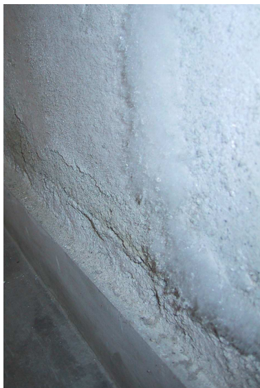
Fig. 19 – Efflorescences and salt damage on a lime-plaster/ paint system, at a corridor (2003-12-04)
