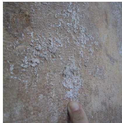
Fig. 12 – Efflorescences on stone (2004-01-06)
