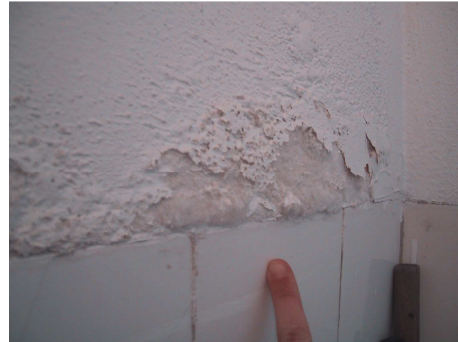
Fig. 23 – Efflorescences, blistering and detachment of the WC "plastic" paint (2004-01-06)
