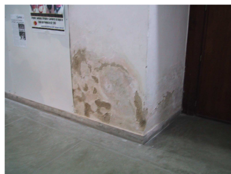
Fig. 14 – Damaged lime plaster/paint system at a corridor (2003-09-11)
