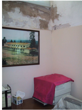
Fig. 24 – Scouts secretary: salt damage on plaster (2003-09-11)
