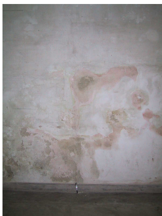
Fig. 13 – Damaged lime plaster/paint system at a corridor (2003-12-04)
