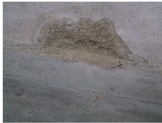
Fig. 18 – Sanding and crumbling of lime-plaster/paint system at a corridor (2004-01-06)
