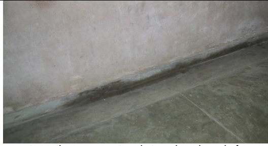
Fig. 21 – Moisture spots on the pavement and stone baseboard of a corridor (2004-01-06)
