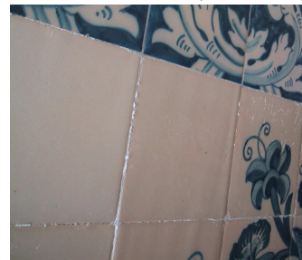
Fig. 10 – Efflorescences on ceramic tiles joints at the entrance stairs (2003-09-11)
