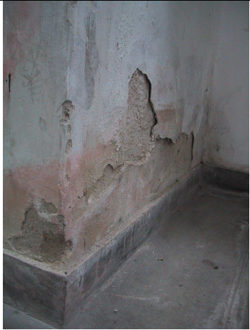
Fig. 15 – Damaged lime plaster/paint system at a corridor (2003-12-04)
