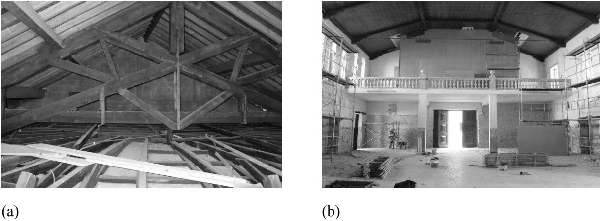
Figure 2. Salesiano's Church: (a) view of the roof structure (example of the existing main trusses), and (b) localization of the choir-organ and its proximity to the ceiling.
