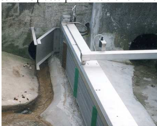
Figure 4-2: Vertical mounted CSO screen type RSW, as retrofit in a existing stormwater treatment work, ROMAG AG - Combined Sewer Overflow Screens for Overflow Structures, Water-Technology.net
