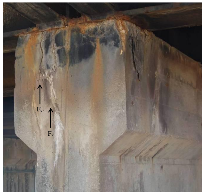
b) Fissura vertical
