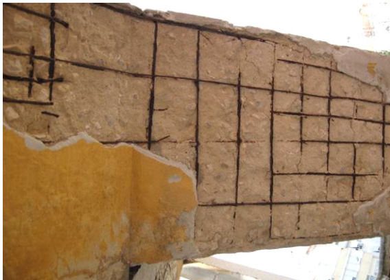
Figure3: Deterioration of landing (underside)
