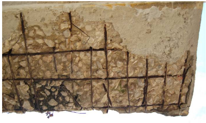
Figure 4: Deteriorated concrete in the final landing
