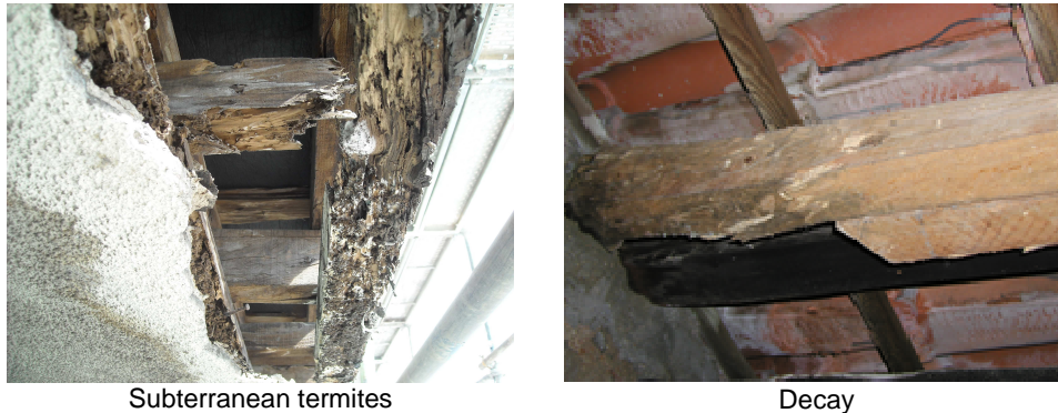
Fig. 3 Biological decay by subterranean termites and wood-decay fungi
