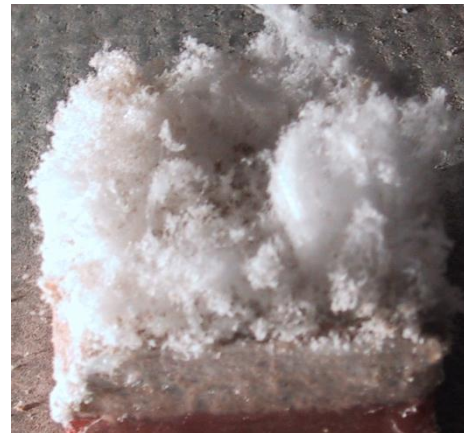
fluffy / hair-like efflorescence
