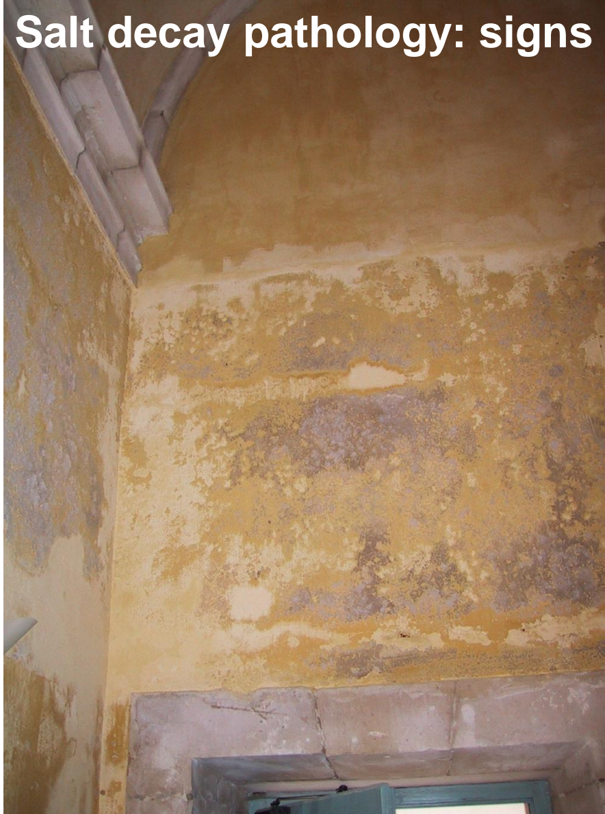
Salt damp and staining
