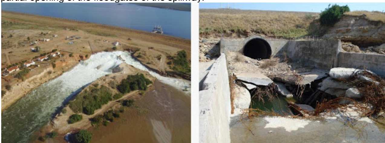
Figure 5 - Accident in the dam (May 2008) and final state of the central area and exits of bottom discharges
