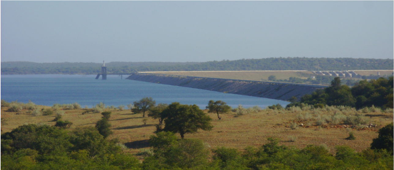
Figure 2 - View of the upstream slope (from the right margin) of the Massingir dam
