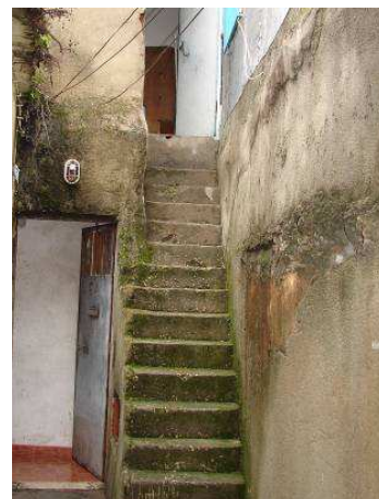
Figure 5. Narrow stairs with uneven development.
