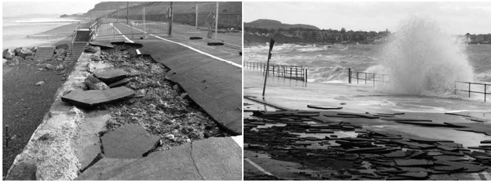
Figure 2. Damage to the existing seawall and wave overtopping at Colwyn Bay
