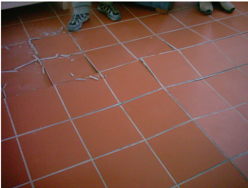
Figure 1: Damaged pavement of the visited upper floor apartment
