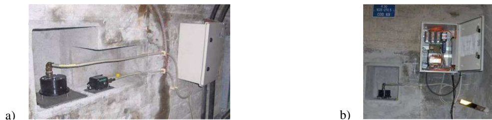
Fig.4 Accelerometers installed at the dam: a) center of the crest gallery b) left abutment.
