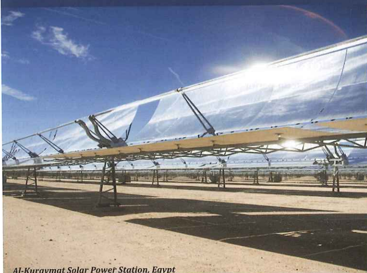
Al-Kuraymat Solar Power Station, Egypt
