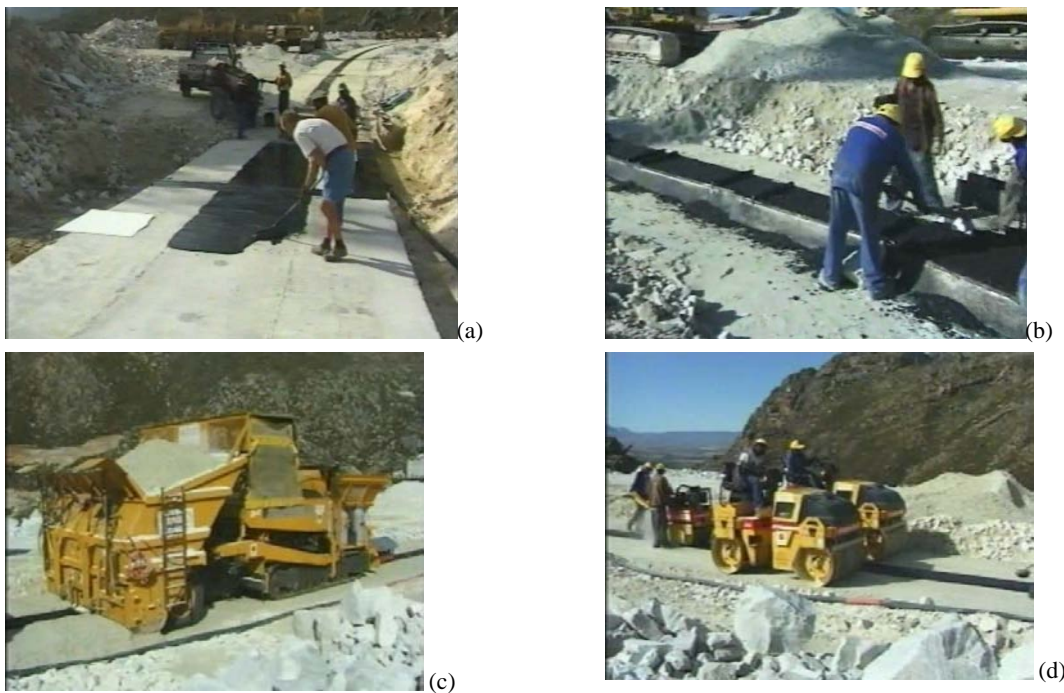
Figure 1 – Illustration of Some Constructive Details: (a) Application Of The Bituminous Mastic Layer; (b) Manual Placing Of Bituminous Concrete; (c) Working Paver; (d) Final Compaction Of Core And Transition Zones (adapted from Kolo Veiddekke, 2008).
