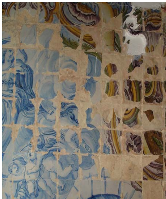
Figure 3: Generalized decay of an interior panel (Igreja de Jesus, Setúbal).
