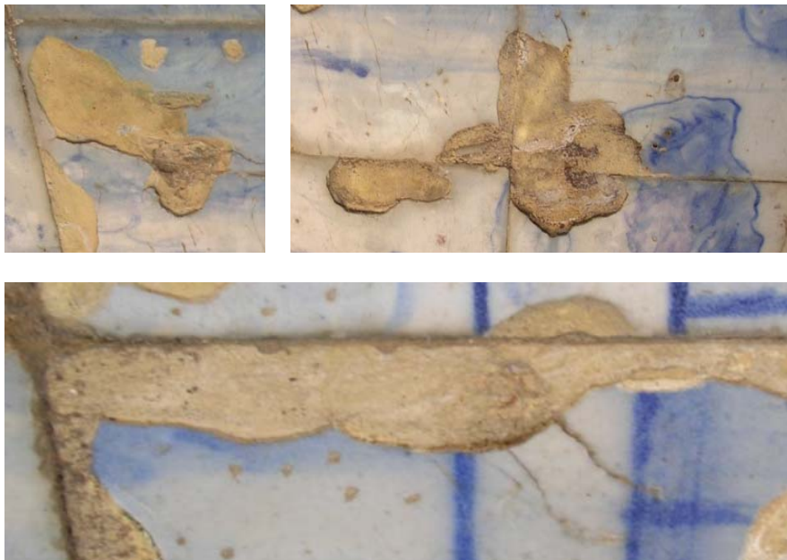
Figure 27: Glaze delamination in azulejo panels located in the upper cloister at NMAz.
