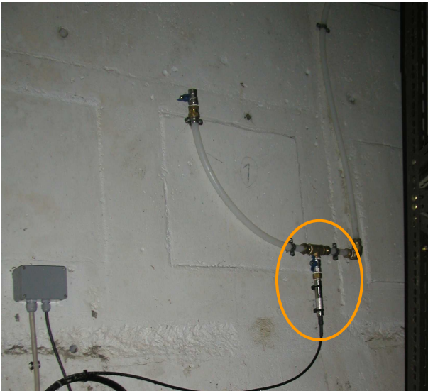
Fig. 6: Pressure cell in a hydrostatic levelling system
