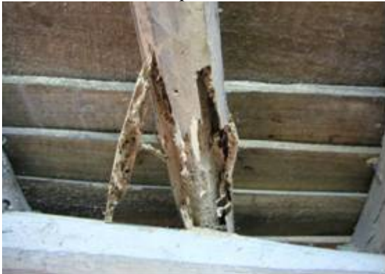
Fig. 5: Detail of the degradation found in a beam of a building in Ponta Delgada
