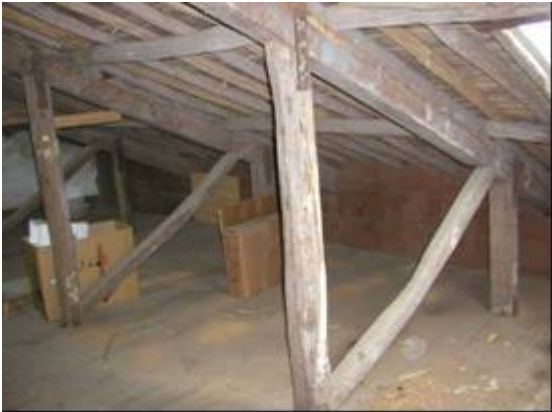
Fig. 4: Example of an infested structure where rehabilitation is still possible
