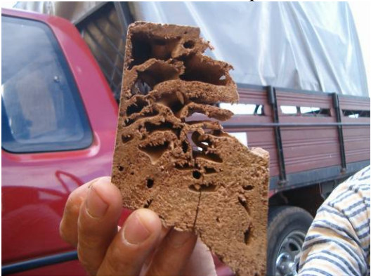
Fig.6: Detail of the degradation found in a roof beam of a building in Angra do Heroísmo (Photo: PestKill Lda.)
