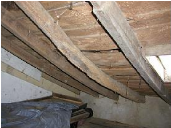
Fig. 3: Example of an heavy infested structure close to rupture
