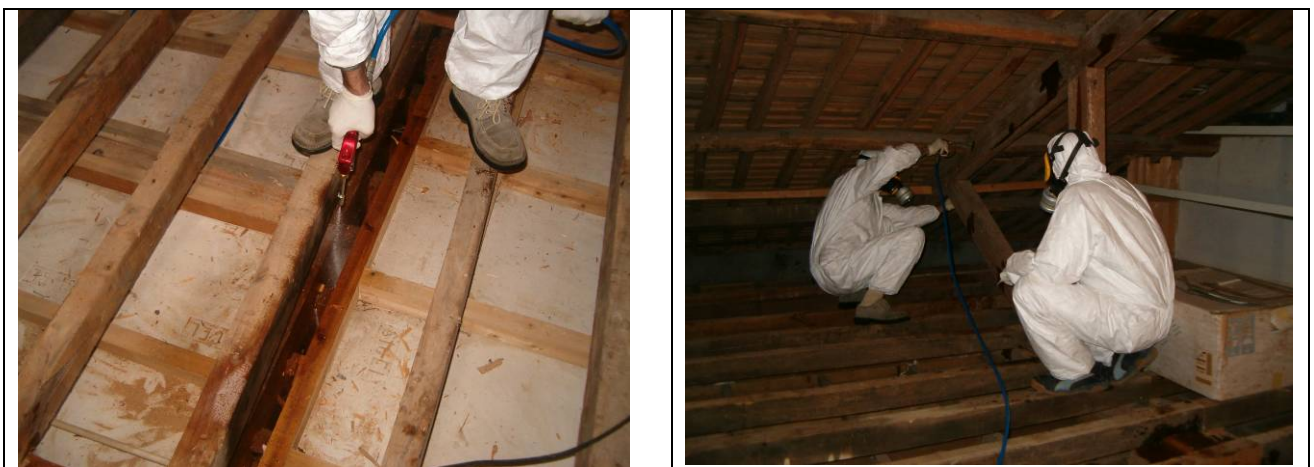
Figure 10: Details of the application of a chemical treatment by aspersion (Photo: PestKill Lda.)
