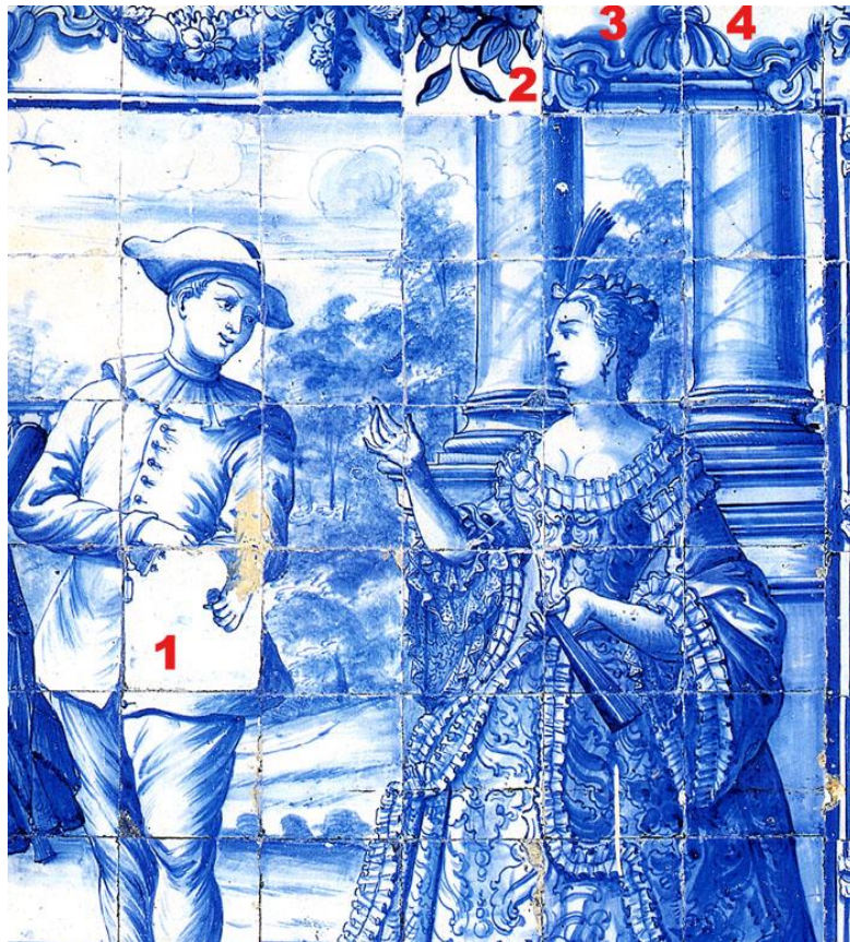
Figure 6- Panel with four missing azulejos reintegrated with replacements at an undetermined date [4]
