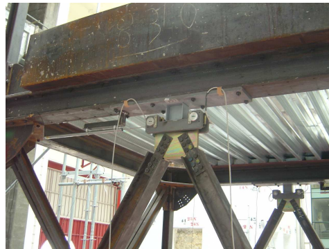
Figure 15: View of Dorka shear panel devices.
