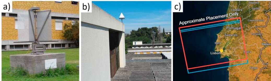
Fig. 2. (a) Corner reflector installed in LNEC complex; (b) GNSS system installed in LNEC complex [5]; (c) Sentinel data layout.
