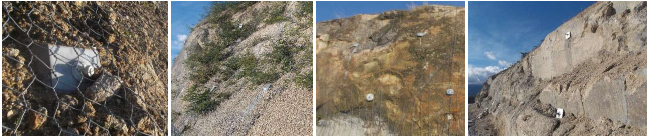
Figure 2. Examples of slope stabilisation in granitic rock masses that have different weathering levels and joint patterns.
