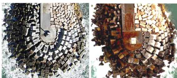
Figure 13: Head of Ericeira breakwater. Two orthomosaic extracts with five years of difference are shown.
