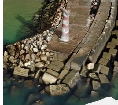
Figure 22: Meshes of Faro-Olhão west breakwater show the movements of the blocks.
