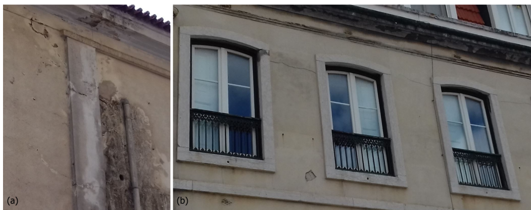
Figure 14. Examples of cracks on buildings associated to centimeter-level displacement clusters, in August 2019. Pictures (a,b) correspond to PSs (a,b) in Figure 13, respectively.
