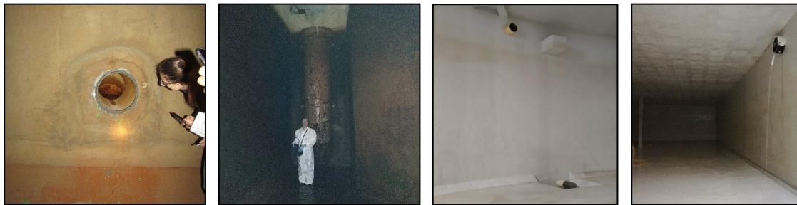
Figure 2.3 – Inlet pipes in water storage tanks.
