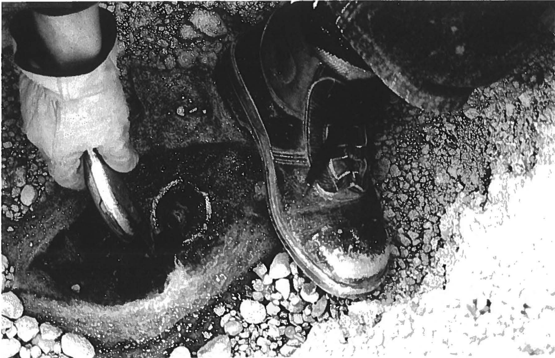
Figure 2. Example of geomembrane damage caused by the seagulls
