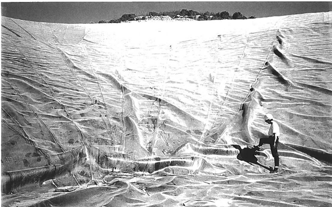
Figure 3. Example of geomembrane waves
