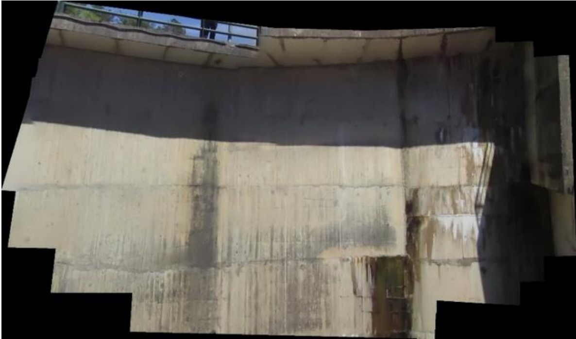
Figure 9 - Orthomosaic obtained with images captured by the aircraft in an operational environment in the dam
