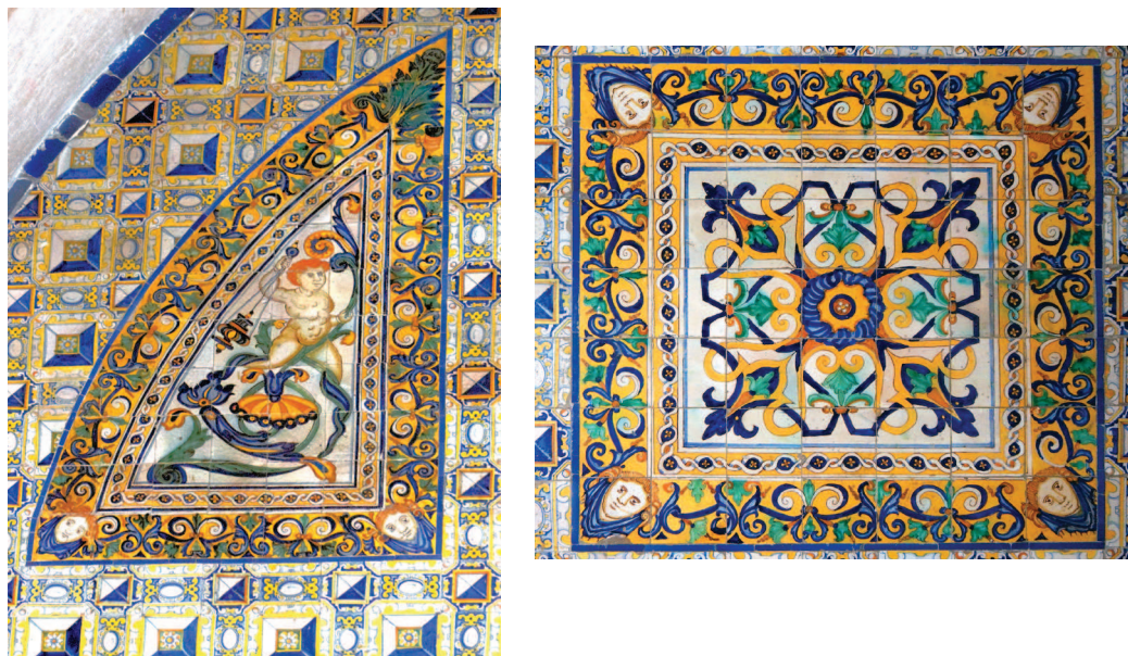
Figure 4. The two sorts of panels set against linings of punta de clavo patterned tiles on the end walls of the transept of Igreja de São Roque. The shape of the corner panel on the left side of the figure shows that it was specifically designed for this particular spot on top of the transept
