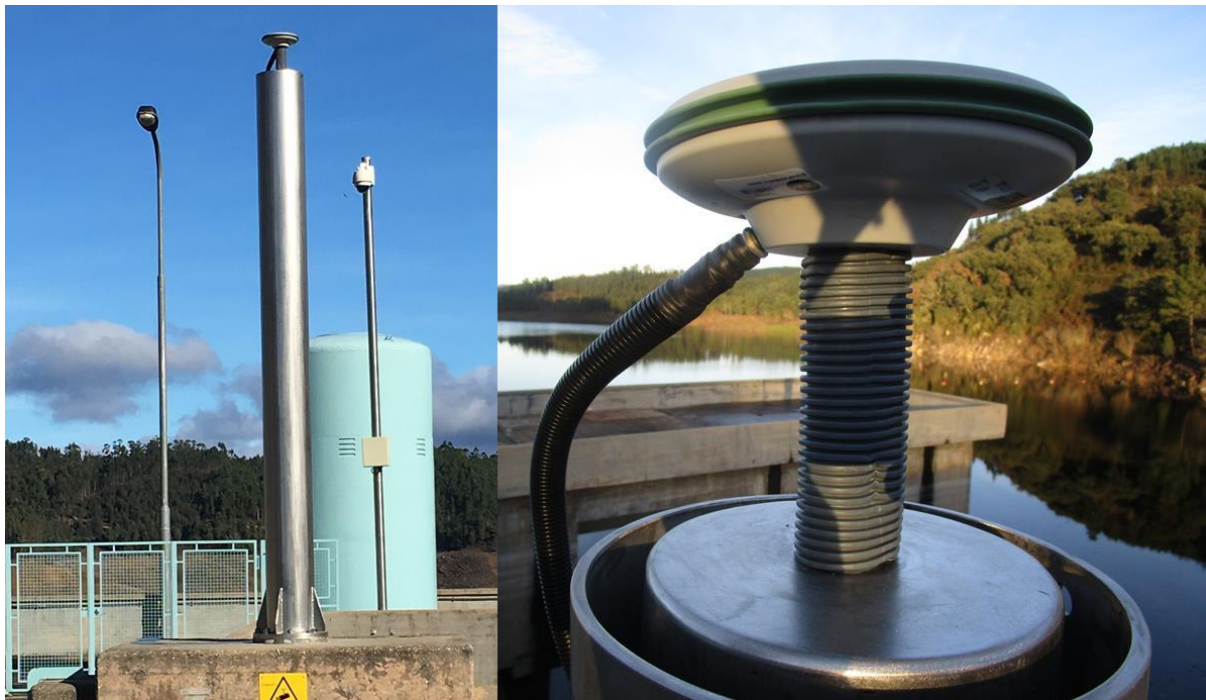
Fig. 4 – The GNSS monument built for the crest of the dam is coaxial dual tubes (on left, a general view, on right, a detail of the monument top with antenna GNSS)
